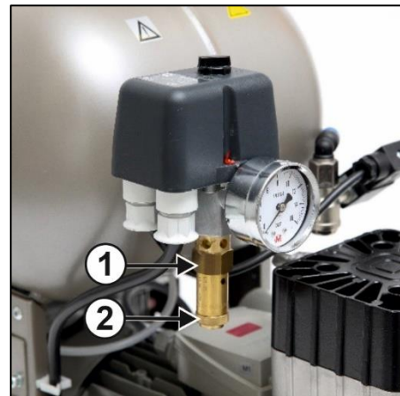
Fig. 13: Check of safety valve
